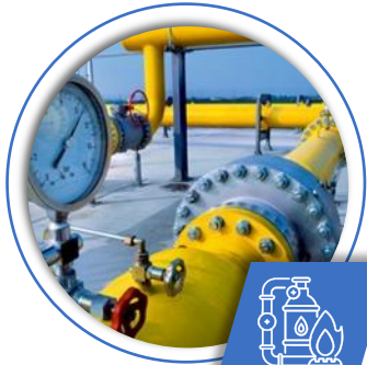
City Gas Distribution
